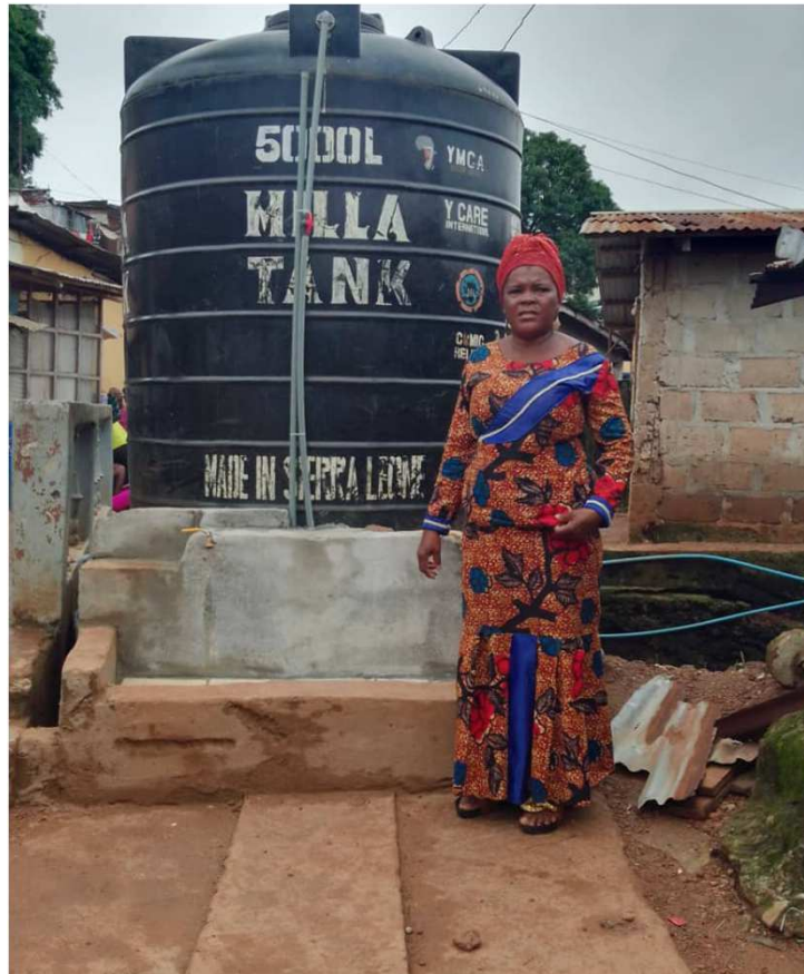
Water tank providing water for Oloshoroh, Freetown, Sierra Leone
